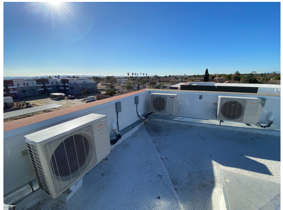
Ducted Minisplits – parapet mounted Condensers
